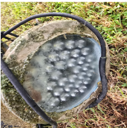
Water in light fixtures
