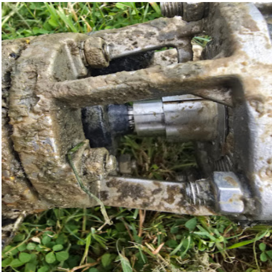
pump & motor shaft is stripped
