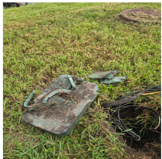
Jbox broken and sunk in
